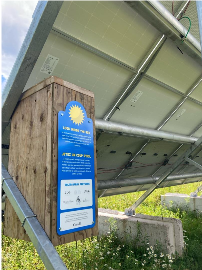
The signage on the inverter box describing how to read the data from the inverter inside the box. Photo: Janie Brooks.
