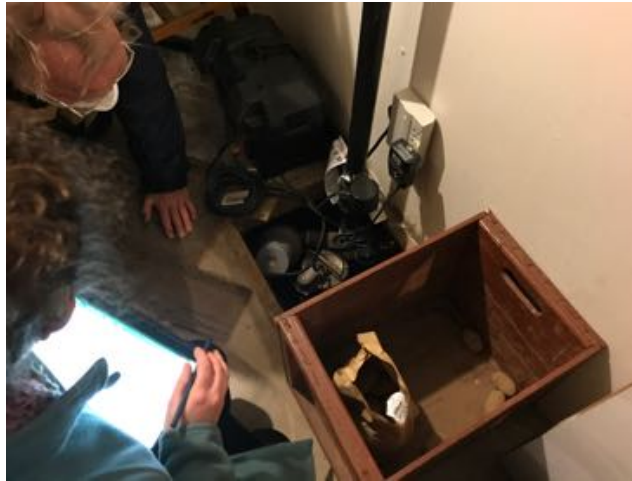
A homeowner and EOS staff examine a sump pump with battery backup and investigate evidence of efflorescence beside it. Photo: A. Marlin
