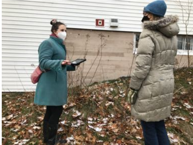
EOS staff and homeowner inspect the landscape grading, foundation walls and windows. Photo: A. Marlin
