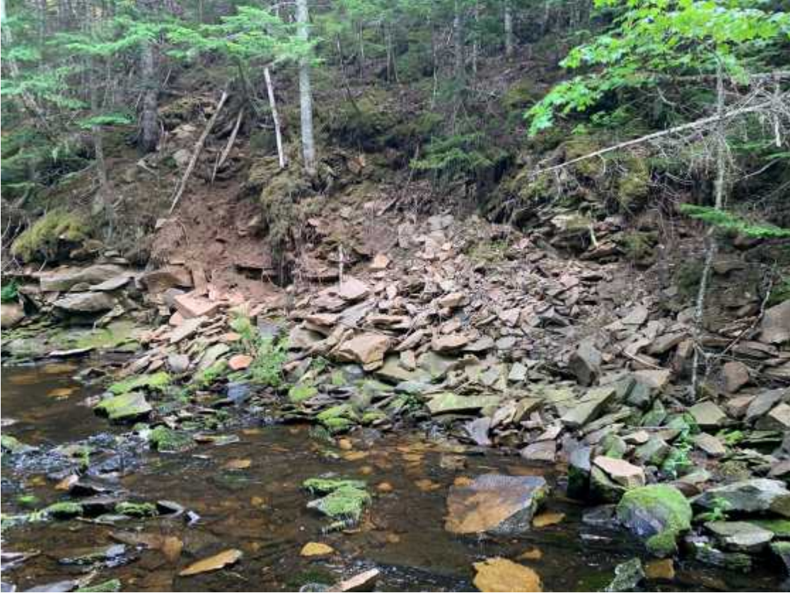
Figure 3: Photo from JB-19 showing an eroded bank
