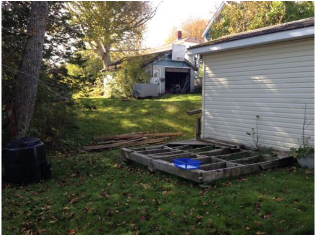
Note: remainder of old deck will be removed and rain garden planted.
