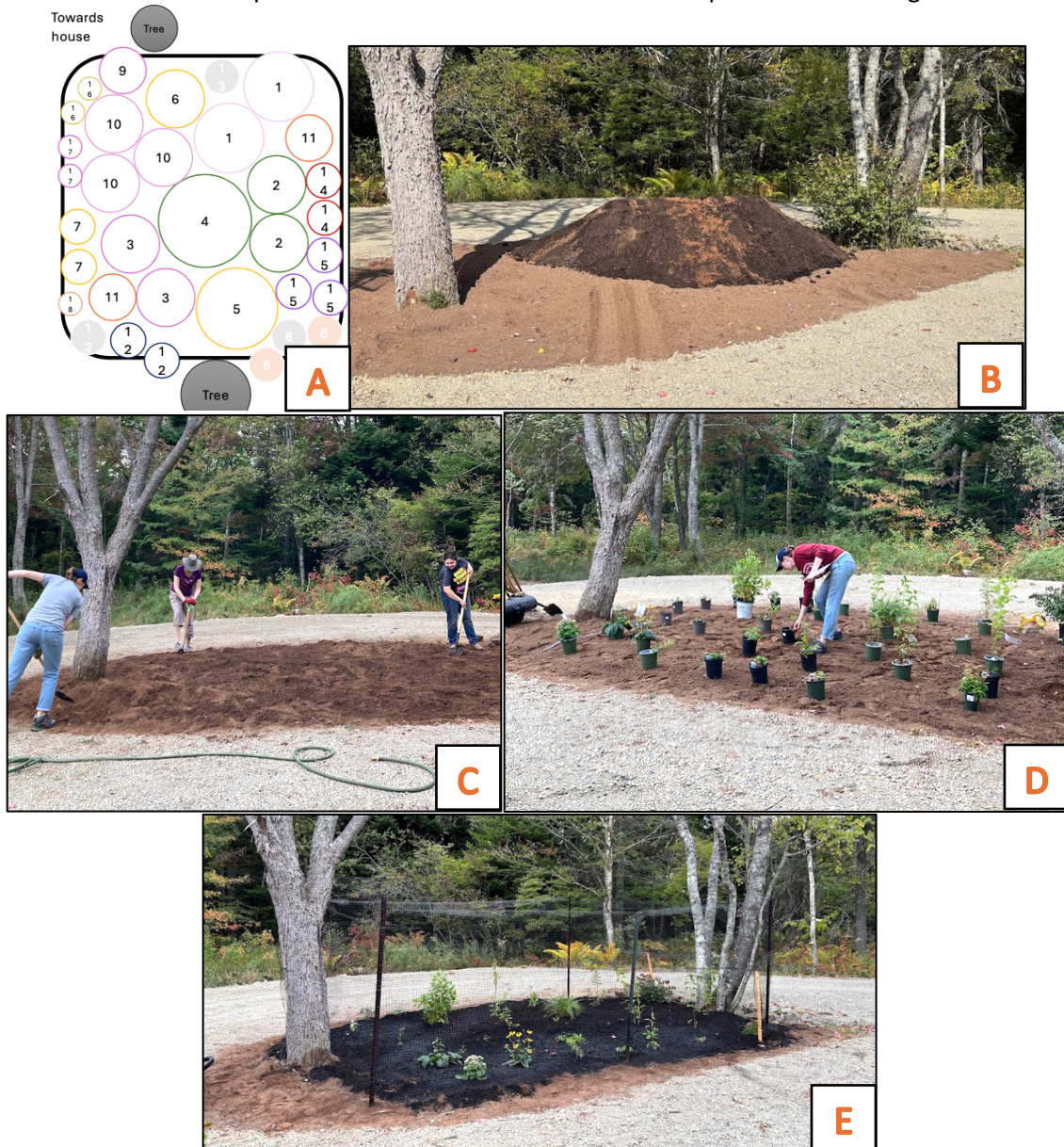
Figure 12: A – Rain garden plant layout and design, B, C, and D – EOS staff and volunteers digging out the rain garden and building up the garden berm, E – The finished rain garden after amending the soil, adding plants, topping off with mulch, and installing temporary deer fencing.
